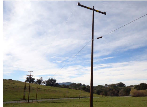
The new steel poles replacing the existing ones have a reddish-brown appearance similar to wood and are known as "weathered steel" poles.
