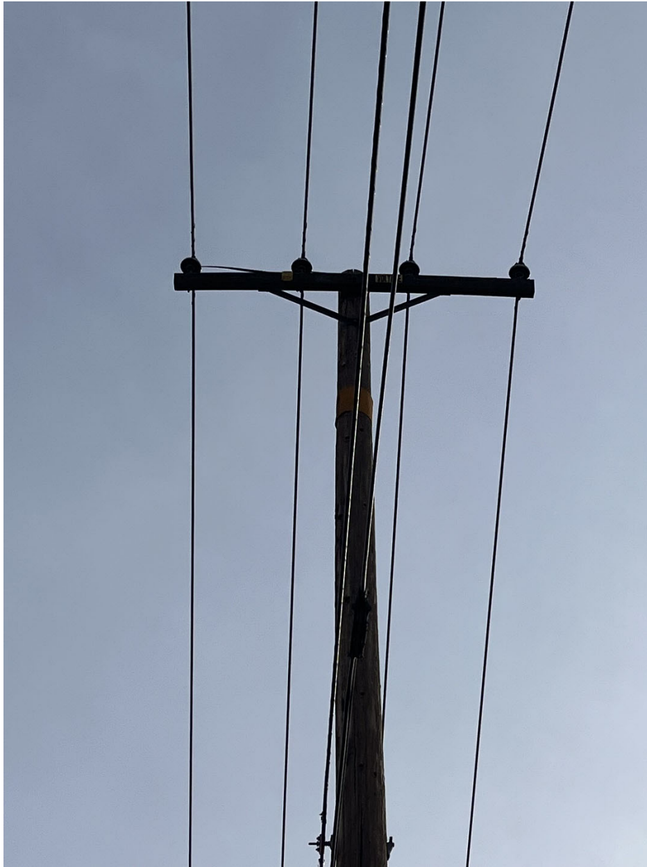
Figure 25 - Item #8 P78880 Damaged Crossarm
