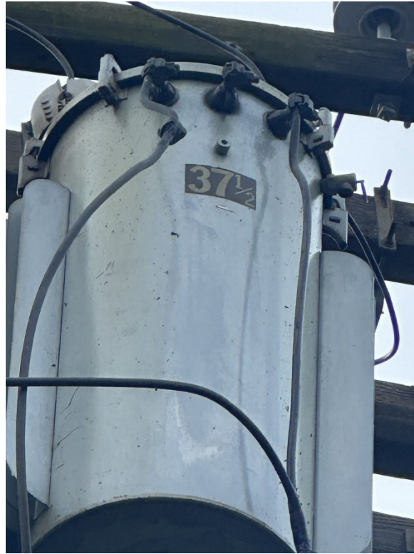
Figure 20 - Item #3 P213996 Leaking Transformer
