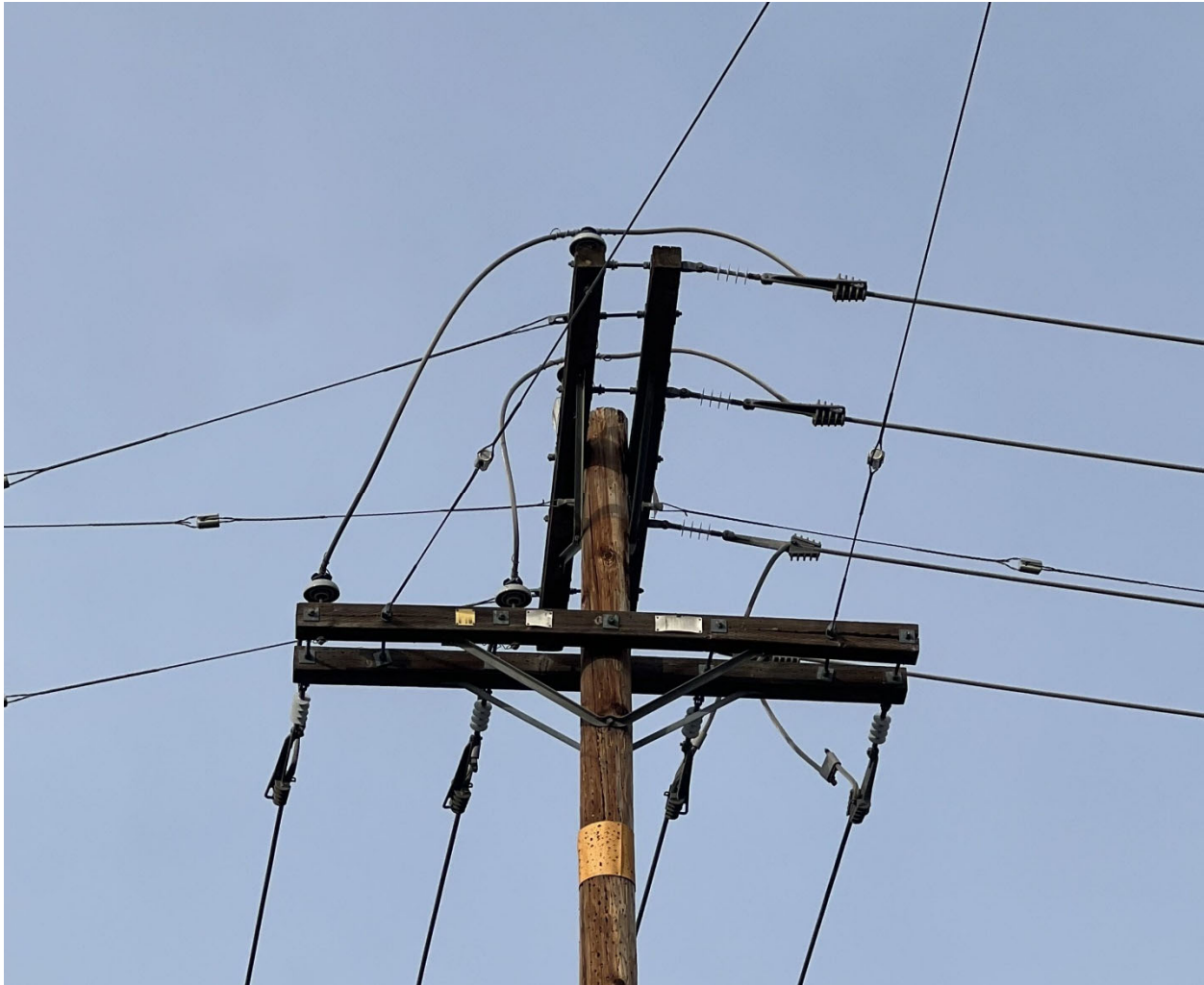
Figure 27 - Item #10 P179023 Damaged Crossarms
