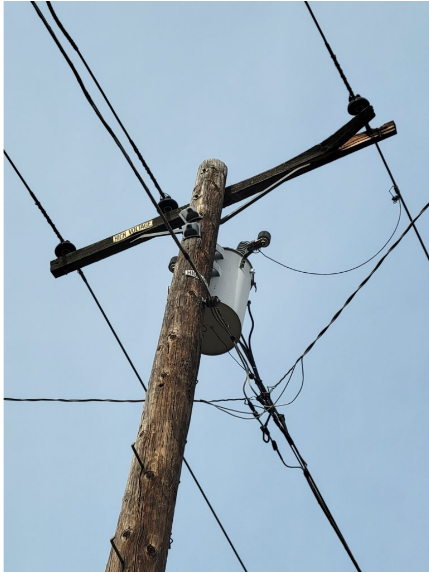
Figure 23 - Item #6 P516439 Damaged Crossarm
