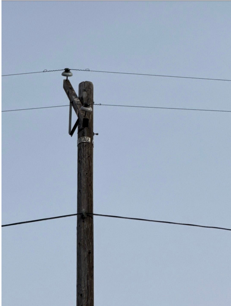
Figure 19 - Item #2 P376436 Crossarm Brace and Bolt Damage
