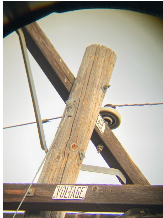
Figure 21 - Item #4 P119515 Damaged Crossarm
