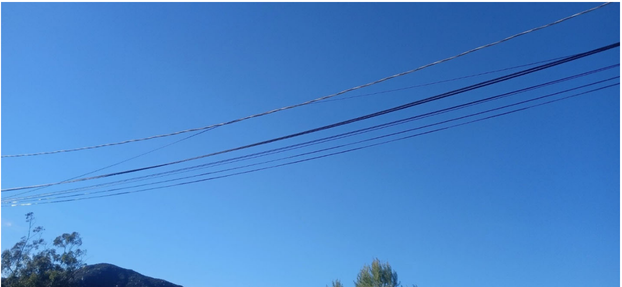
Figure 18 - Item #1 P710840 Telco Lashing
