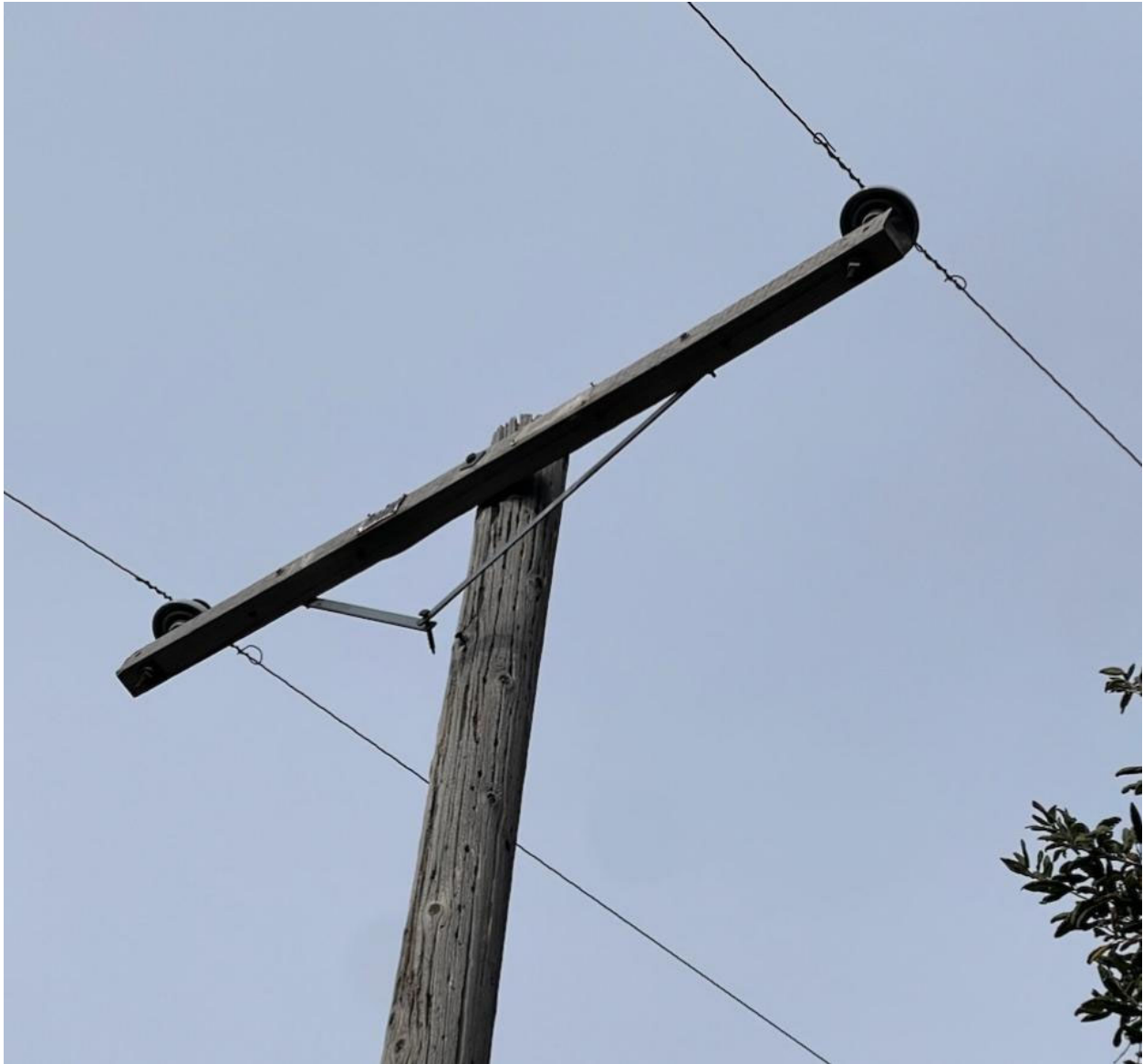
Figure 26 - Item #9 P166012 Crossarm Brace and Bolt Damage
