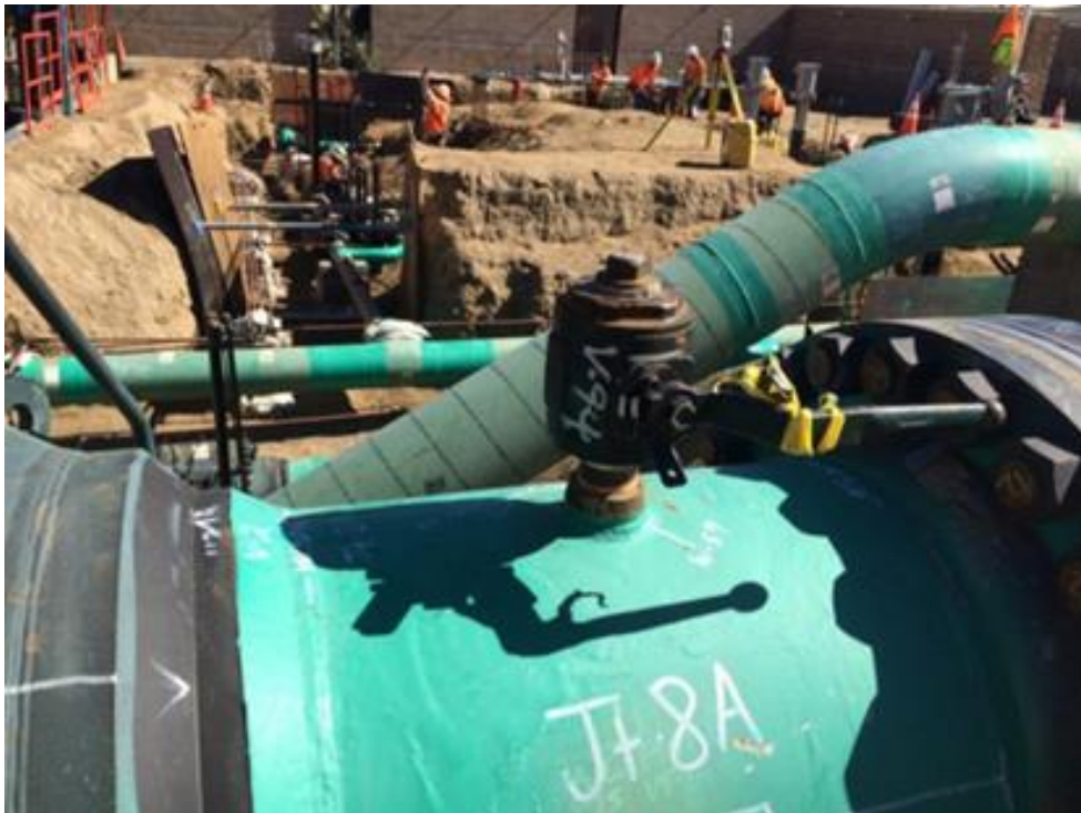
Figure 18: Large Valve Station with Numerous Above-Ground Features
