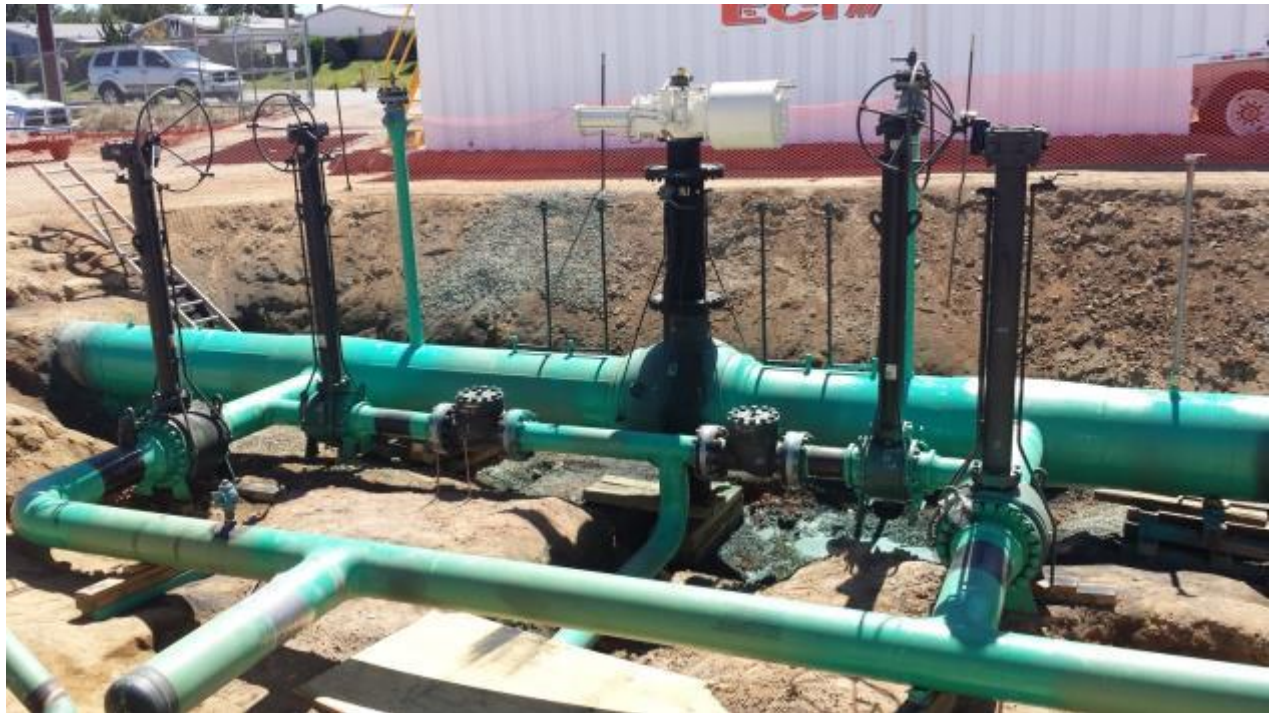
Figure 7: Assembly for L235W at Palmdale Tap: 30" MLV 235-215.22-0 shown with new actuator (in white) along with ■ bridle valves to and check valves to SL 44-654; ■ blowdown valves are also shown.
