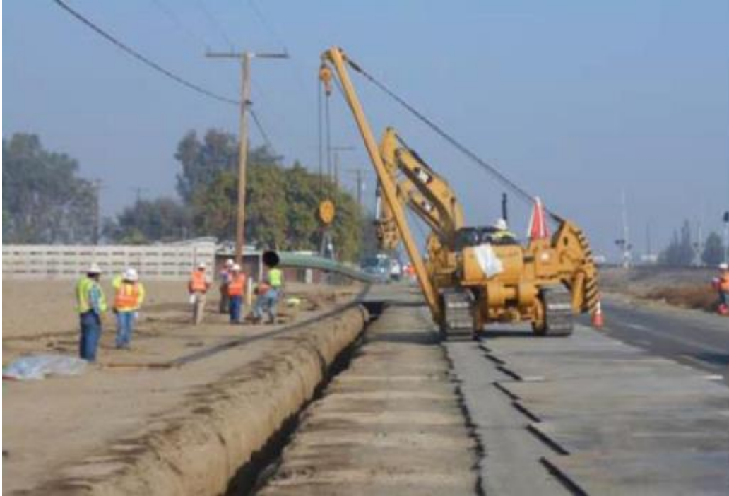
Figure 3: Placing Pipe in Trench with Side Boom Equipment along S I Street and plates to protect asphalt
