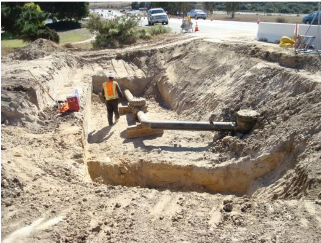
Figure 16: Traffic Control Activities and Exposed Pipeline Along Harris Grade Road (Old Highway 1) In Section 2
