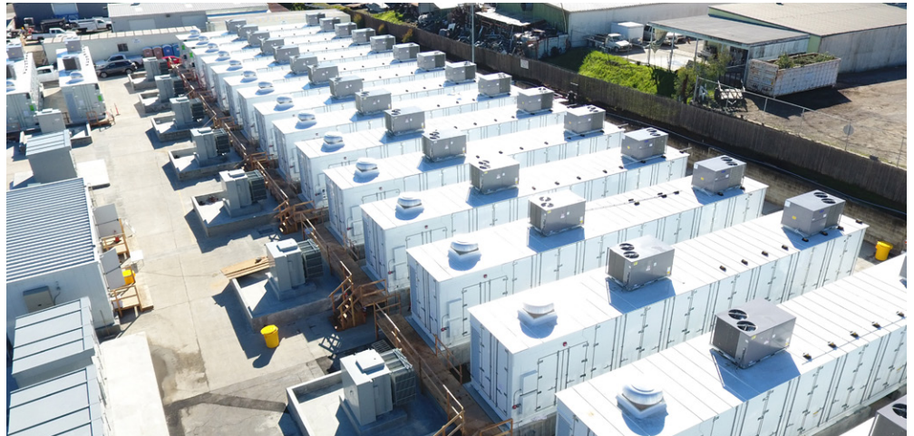
Escondido Battery Energy Storage System project
