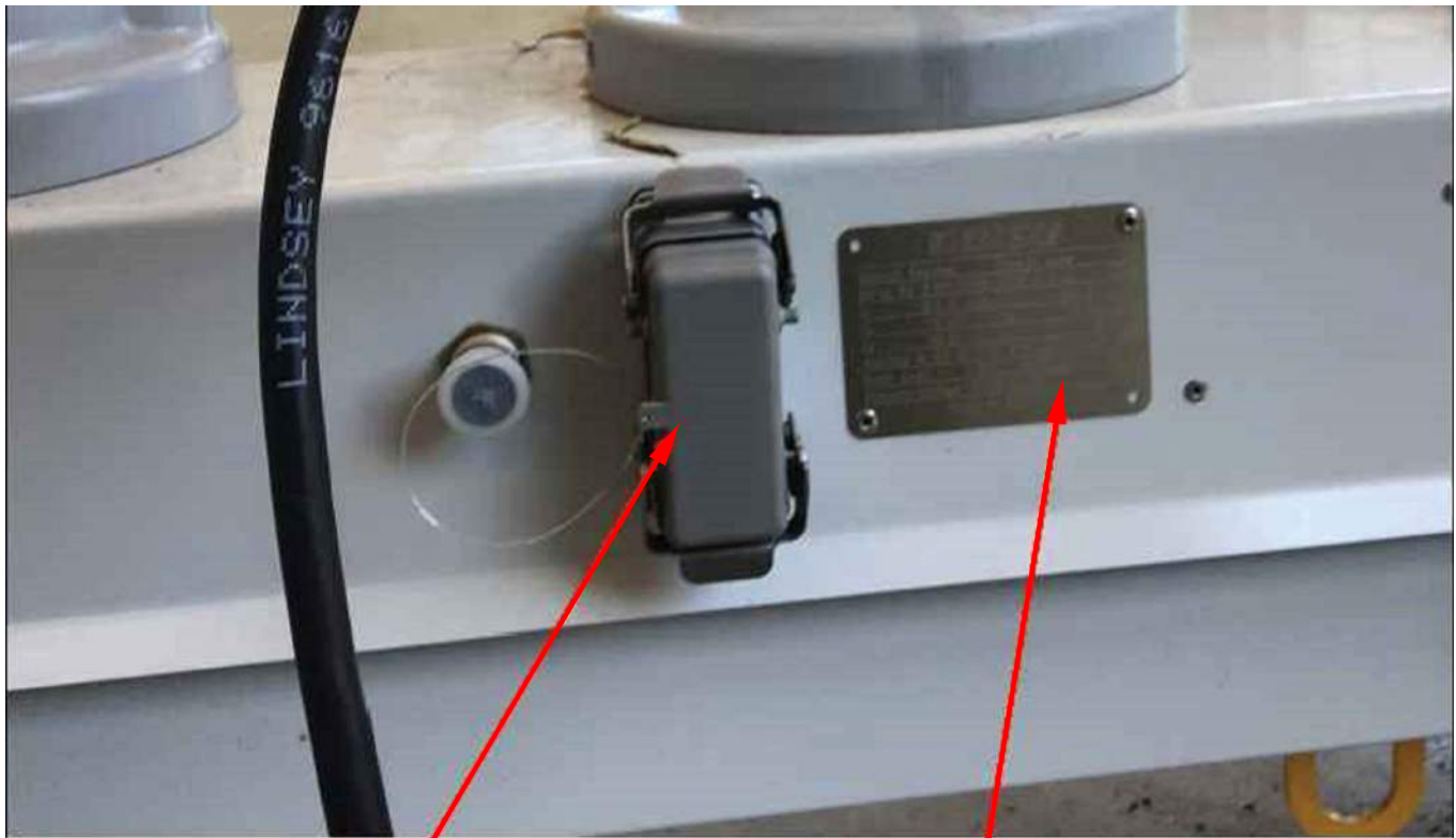
CONTROL CABLE CONNECTOR
