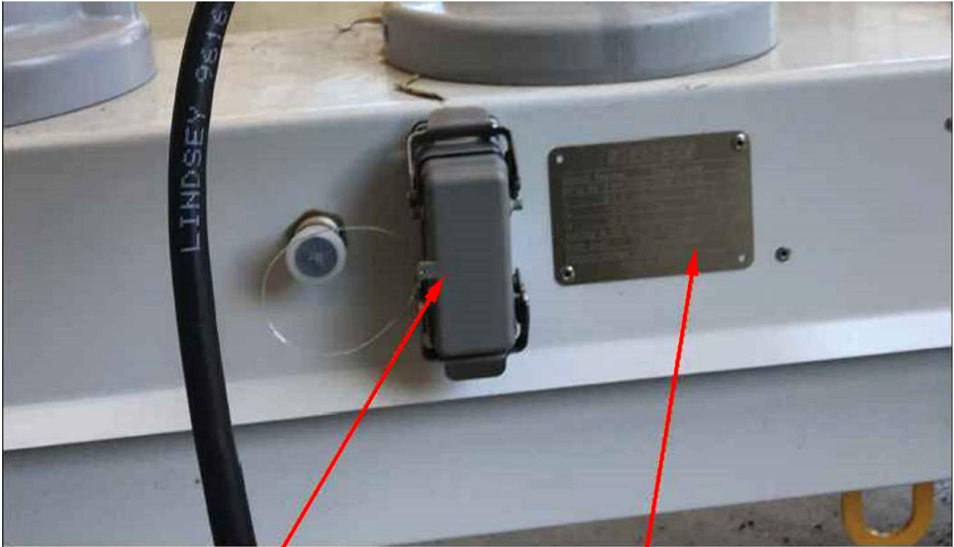
CONTROL CABLE CONNECTOR
