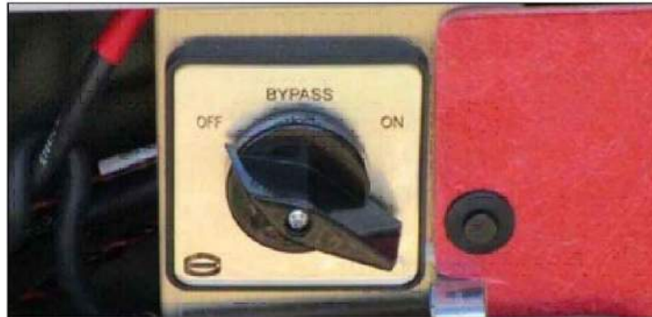
FIGURE 5 BYPASS SWITCH (E)
