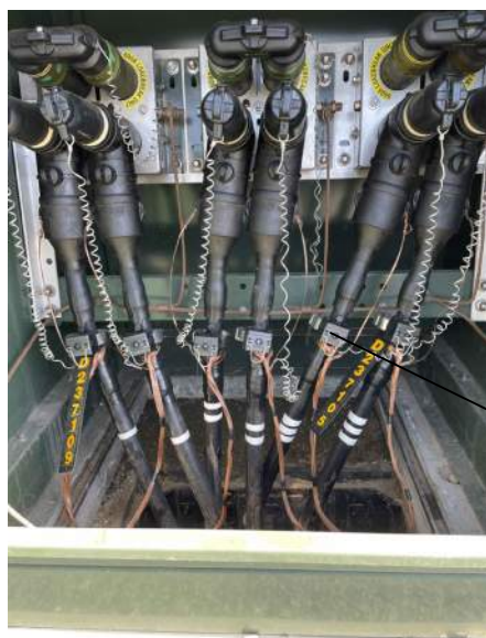
FIGURE 2 WITH LOAD TRACKER FAULT INDICATORS
