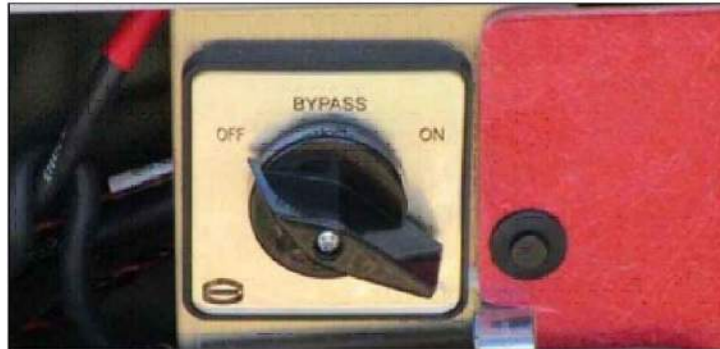
FIGURE 5 BYPASS SWITCH (E)
