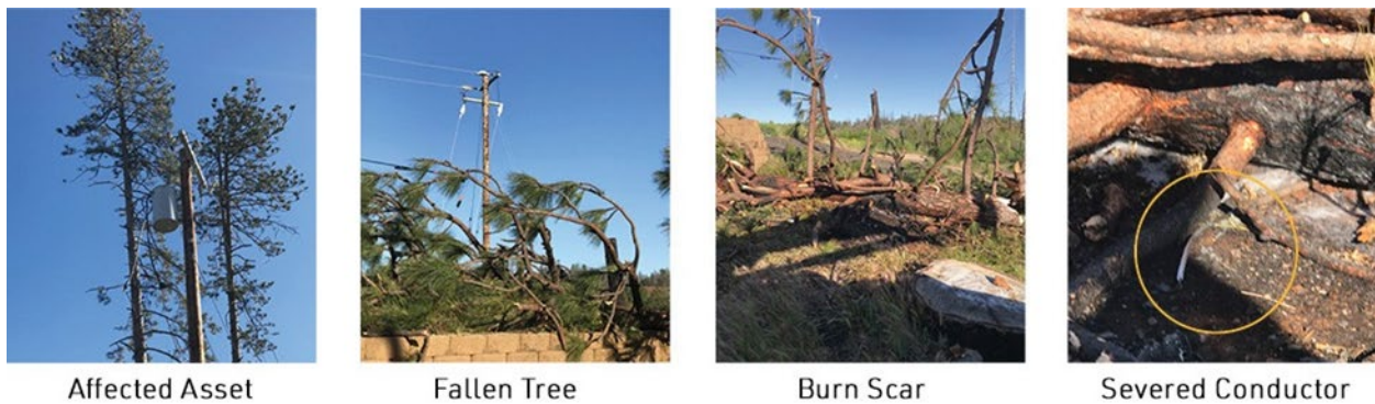
Figure 2: PG&E Covered Conductor Effectiveness – Example 1
