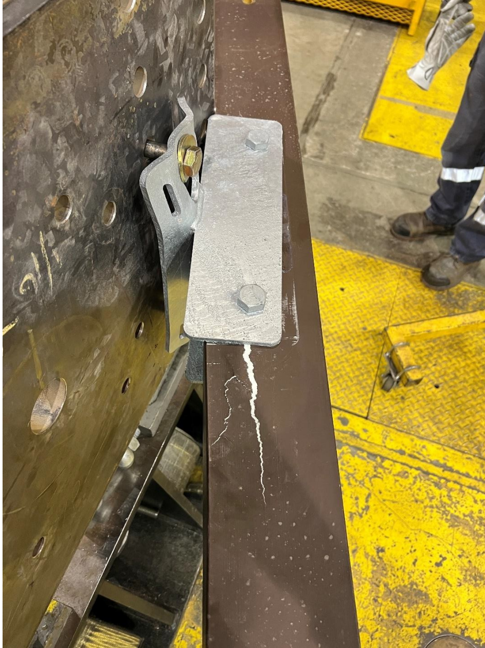
Figure 6-17: Sample 4.1 – Failure Location
