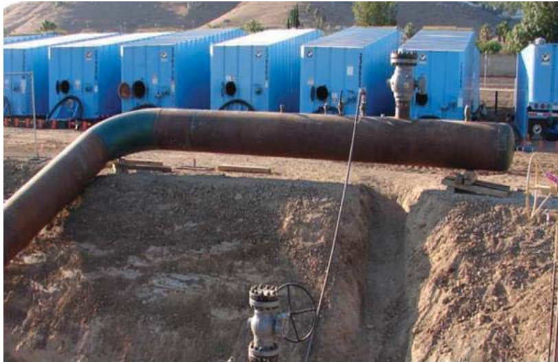
Figure 26: Water Tanks and Test Head
